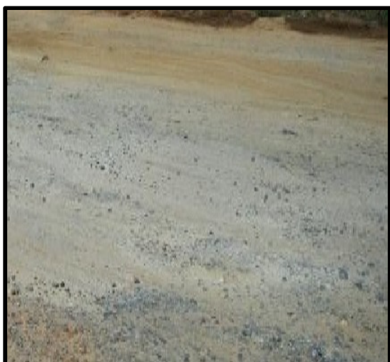
Figure.4.1 Existing Condition of road Due to Bad Drainage
