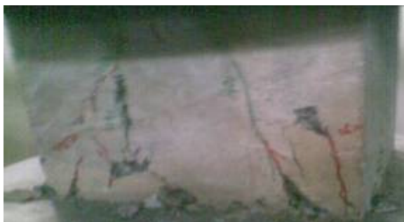
Fig. 7.2 Vertical Cracks leading to Column fragments
