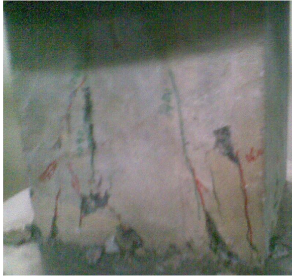
Fig.10 Vertical Cracks leading to Column fragments
