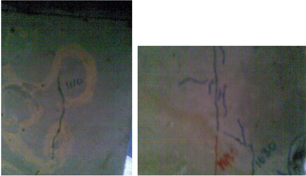
Fig. 8 Initiation of Crack and its propagation at higher stress levels
