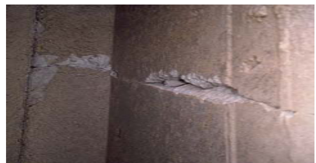
Fig. 1: Horizontal crack at lift joints(left: crack at upstream face; right: crack in web of buttress at downstream face of the dam)
